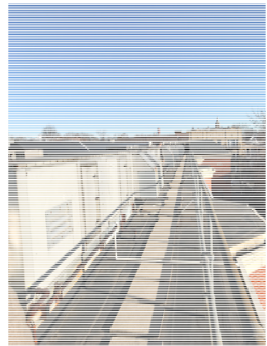
Figure 6. Bethune HVAC Equipment
